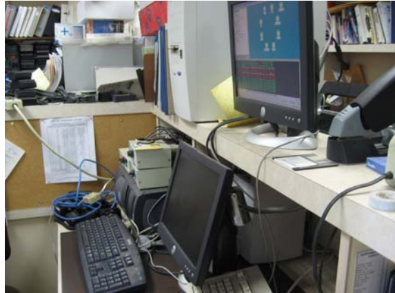
Motorola Alarm System Trunking System
