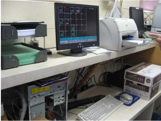
Site Alarm Panel for Radio Sites
